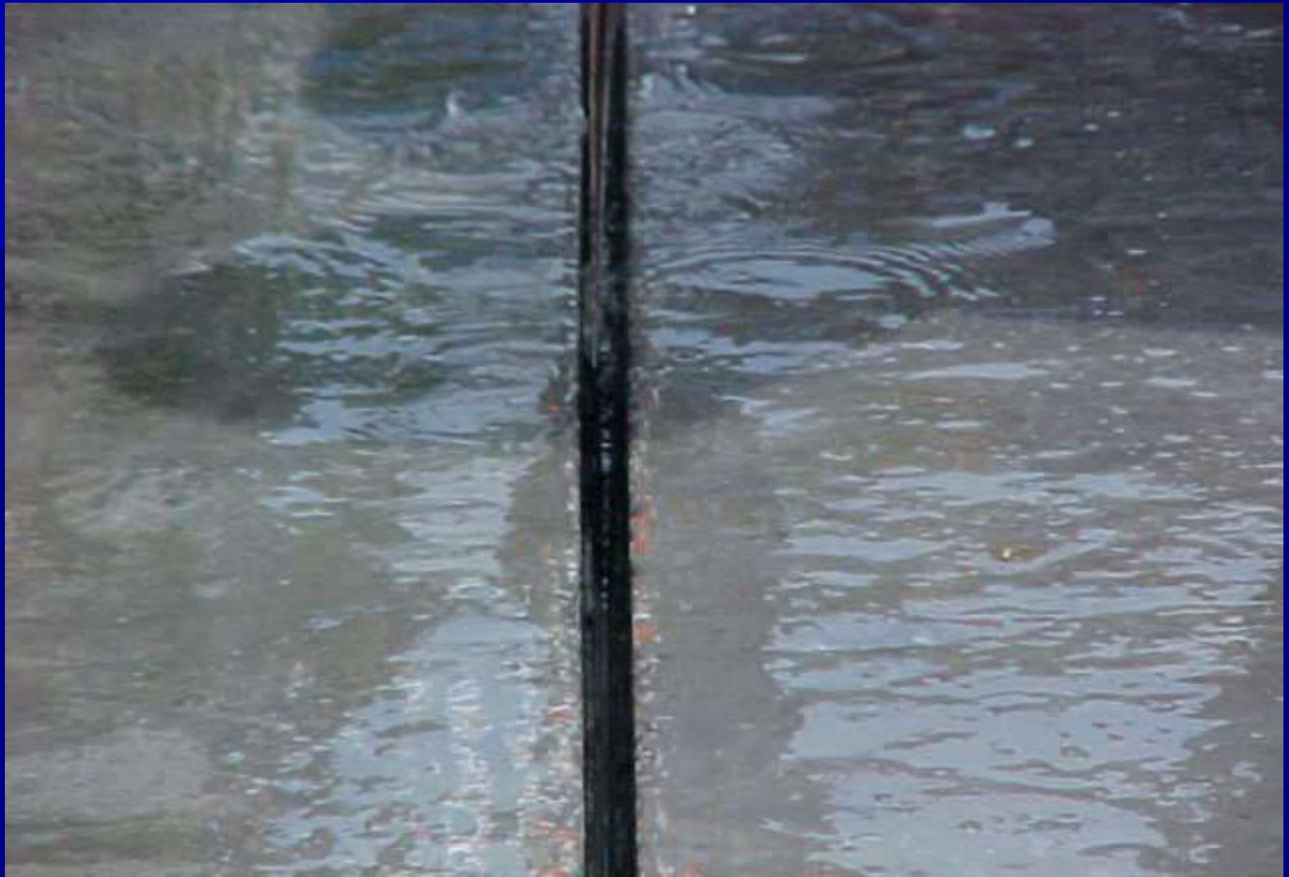
Widened Groove after 14 days
