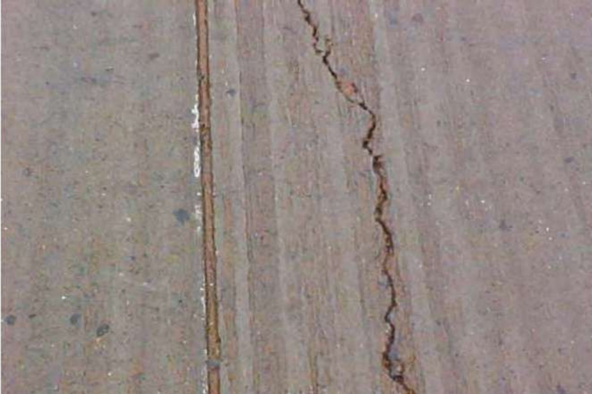
Crack caused by late joint sawing
